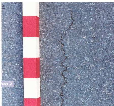
FIGURE 2.1. Fissure transversale : fissure franche et perceptible [LCPC, 1998]
